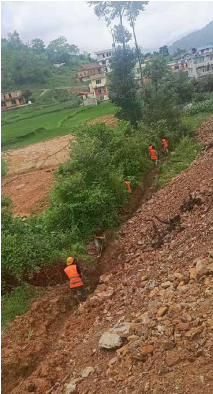
Distribution pipeline, Lele
